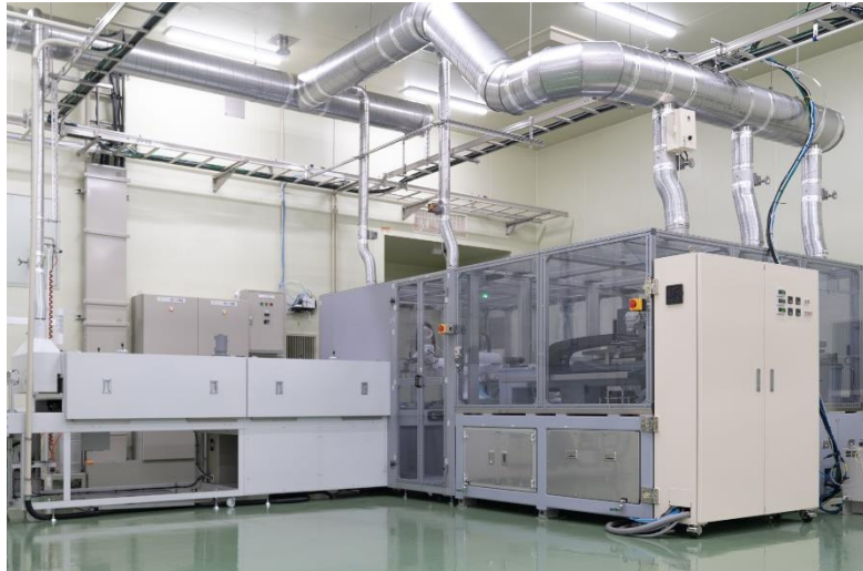
ELP03 mass production machine in operation
